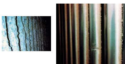
Superheater before and after Innospec's heavy fuel oil treatment
